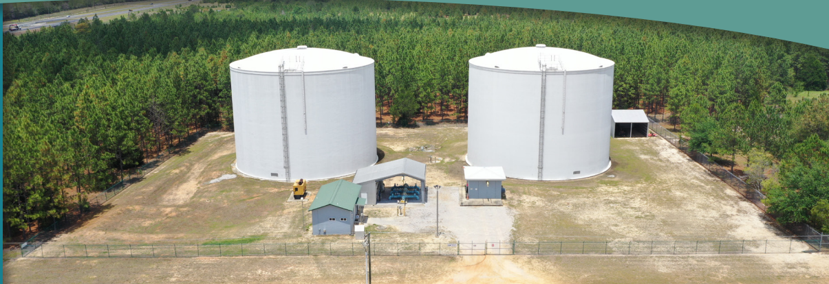
Nokuse Wellfield Water Storage Tanks
